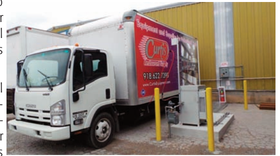
Single refueling station onsite
